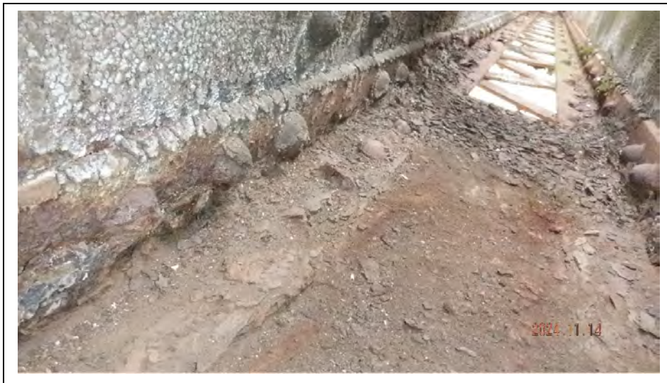
Photo 11: Asset 5104 Span 3 Bottom Chord Section Loss to Interior Angles
