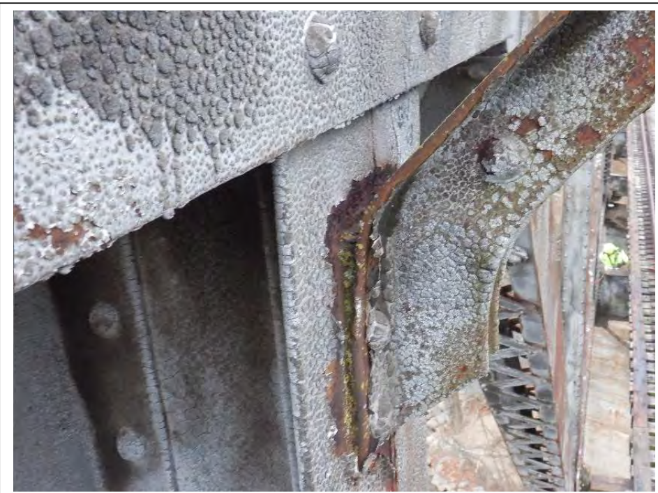
Photo 12: Aset 5104 Span 3 Section Loss at Portal Brace Connection
