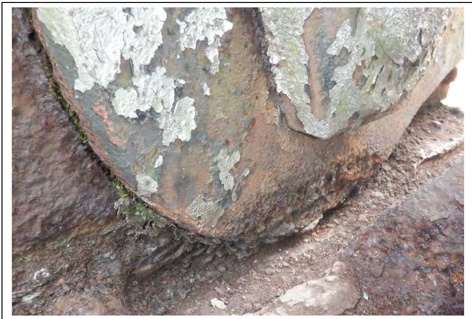
Photo 09: Asset 5104 Typical Eye-bar Section Loss at Connection
