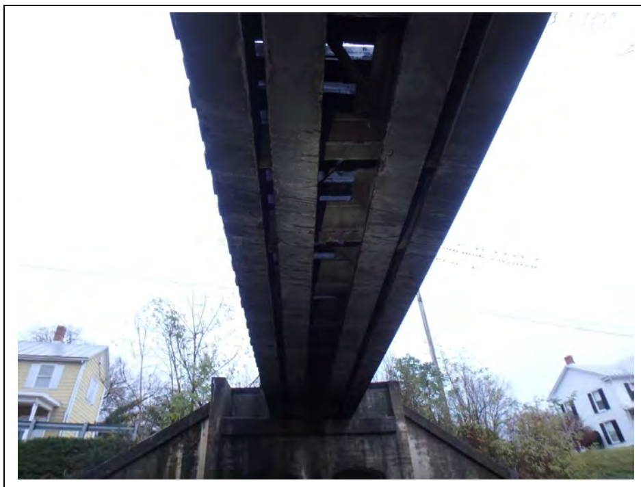
Photo 14: Asset 6141 Diaphragms and Top Lateral Bracing
