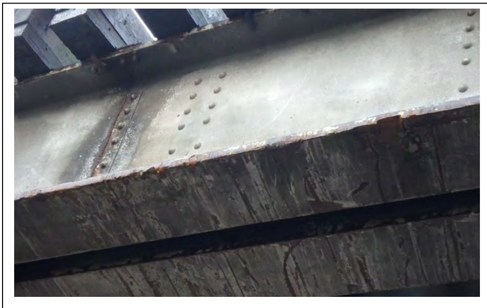
Photo 16: Asset 6141 Impact Damage Bottom Flange
