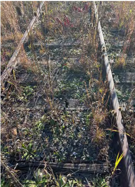
Figure 7 – Fouled Ballast, Jointed 85# Rail, Excessive Tie Deterioration
