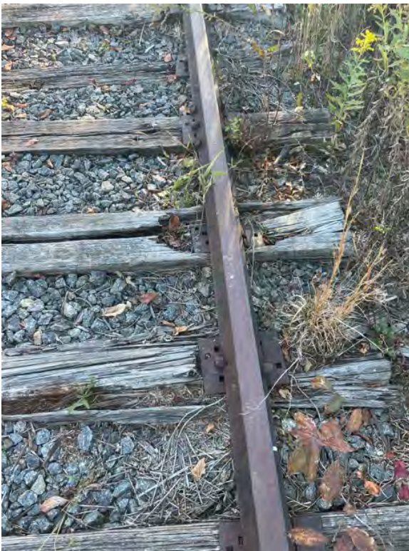
Figure 8 - Poor Crosstie Condition
