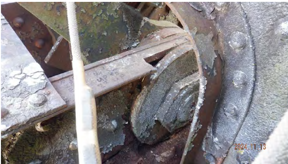
Photo 08: Asset 5104 Span 2/4 Eye-bar Section Loss
