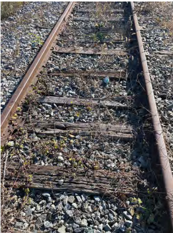
Figure 6 - Poor Crosstie Condition. 100# Rail and OTM in acceptable condition
